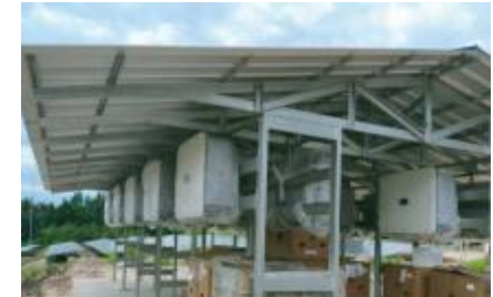
Inverters control panel
